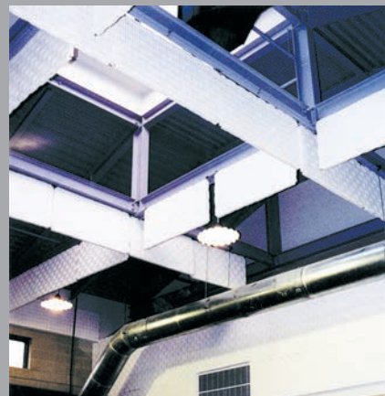
SONEX® One baffles in music room
